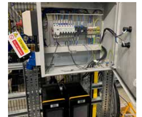
Inside the electrical cabinet for the ITER Vacuum Vessel Pressure Suppression Remote Handling System trials
